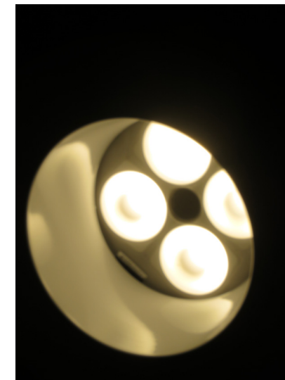
TYPICAL RECESSED CAN FIXTURE WITH LED
