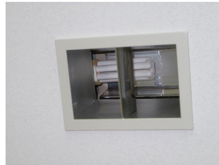
TYPICAL CORRIDOR LIGHTING FIXTURE WITH COMACT FLUORESCENT LAMP
