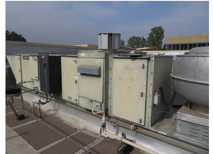
TYPICAL PACKAGED ROOFTOP UNIT
