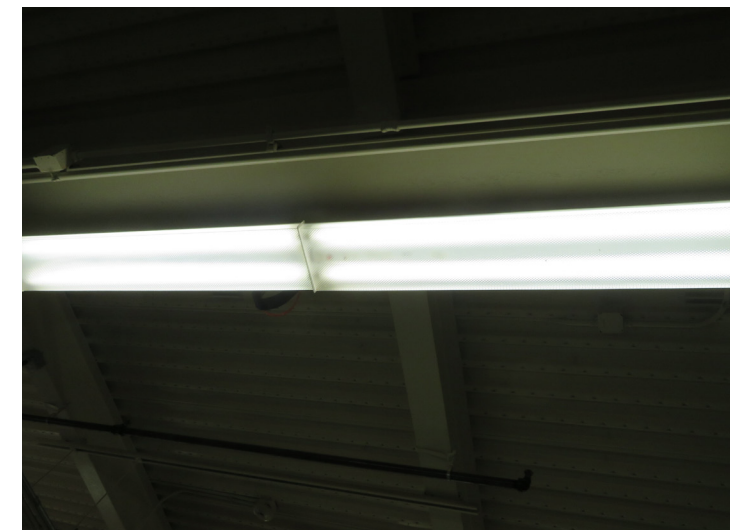
TYPICAL LIGHTING FIXTURE WITH F32T8 LAMPS
