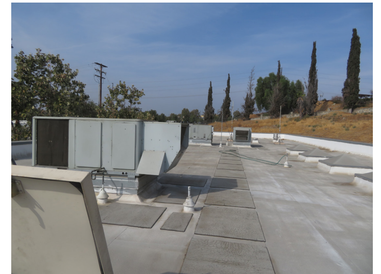
TYPICAL PACKAGED ROOFTOP UNIT
