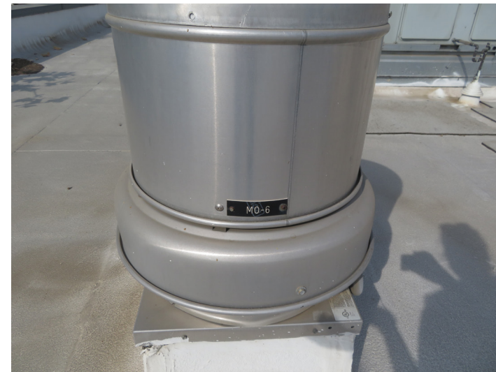
TYPICAL EXHAUST FAN
