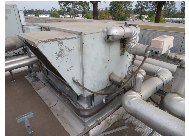
AIR HANDLING UNIT WITH CHILLED WATER CONNECTION
