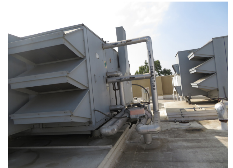
TYPICAL AIR HANDLERS WITH CHILLED WATER CONNECTIONS
