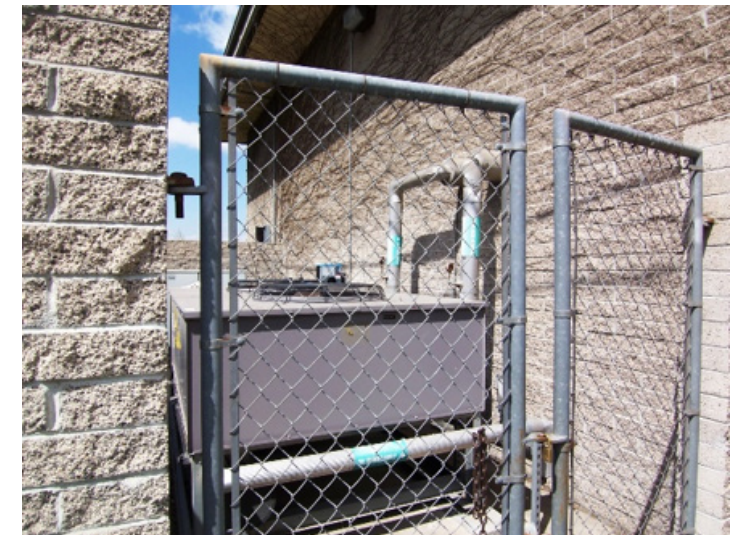
AIR-COOLED CHILLER SERVING BUILDING
