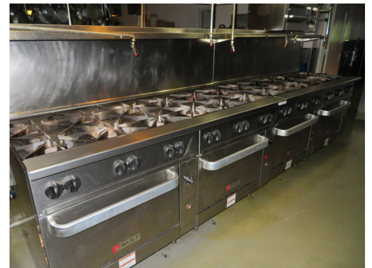
KITCHEN GAS-FIRED STOVE TOPS
