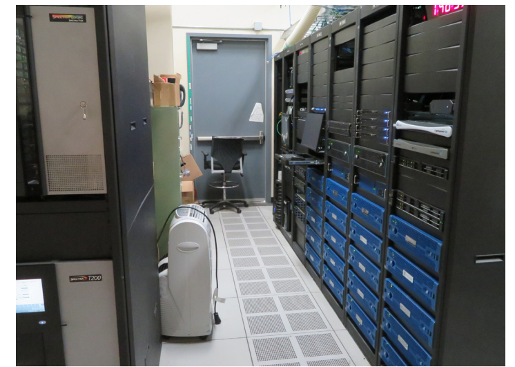
DATA CENTER SERVER RACKS
