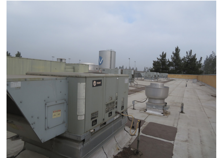
TYPICAL PACKAGED ROOFTOP UNITS
