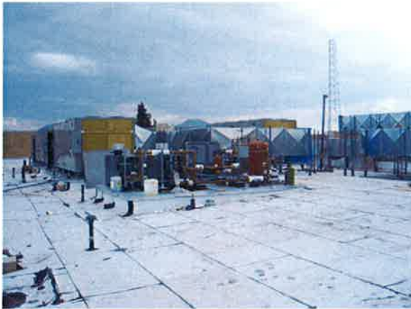
HVAC roof units
