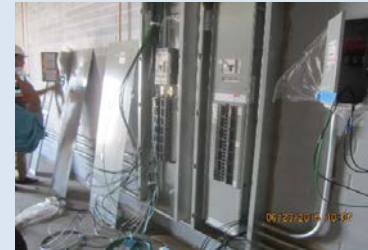
Electrical Panel Wiring
