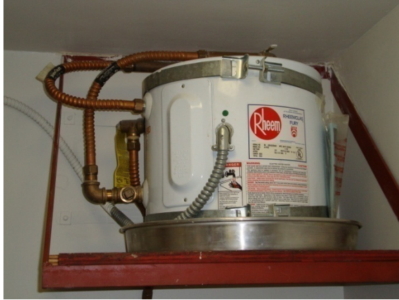
Figure 10 Existing DHW Heaters
