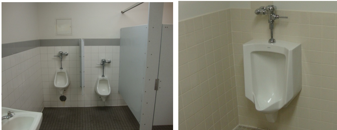
Figure 13 Installations of Flushed Male Urinals at SBCCD
