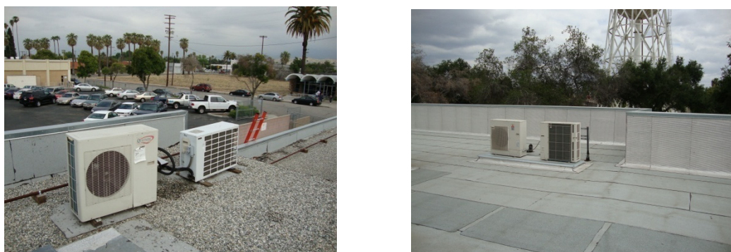
Figure 9 Few Installations of Condensing Units at SBCCD
